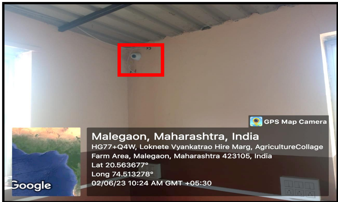
CCTV Camera in Class Room
