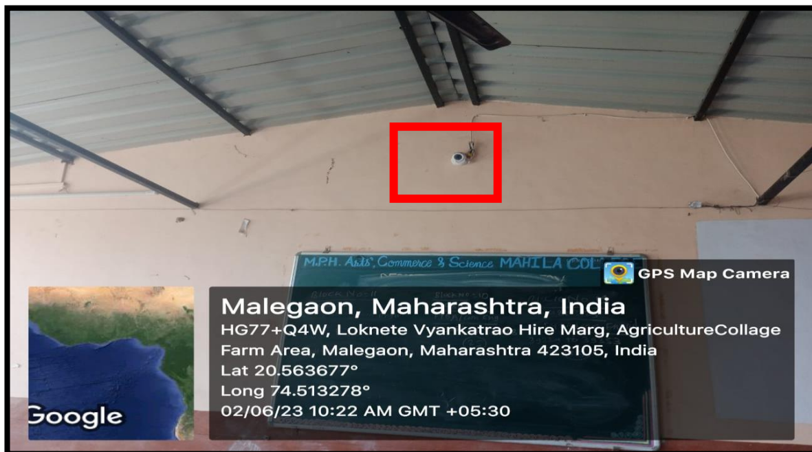
CCTV Camera in Seminar Hall
